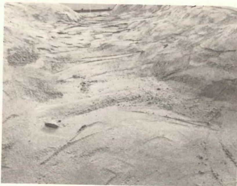
Figure 37.—Eroded material deposited downstream of the spillway in the river channel at STA 1 + 684.0. P801-D-79595.
