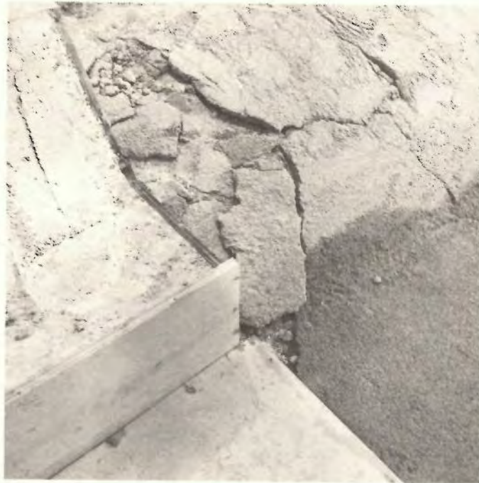
Figure 34.—Erosion at the toe of the spillway apron and along the left riverbank. P801-D-79592.
