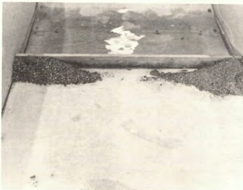
Figure 35.—Deposition of eroded material downstream of the spillway sill. P801-D-79593.
