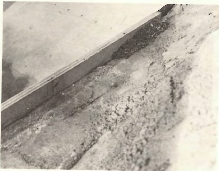
Figure 36.—Eroded material collected behind the left spillway training wall. P801-D-79594.
